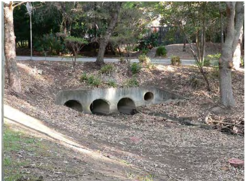
Plate 6: Starting point of the watercourse. The three large pipes connect directly to Greville Street.
